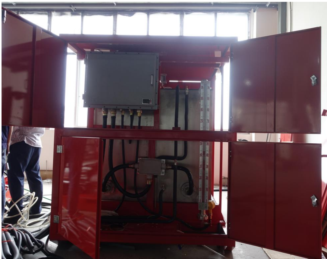
Figure 2.12 Chemical Reagent Storage Skid
